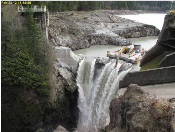
Fig. 4. Removal, in 2014, of largest dam in the United States to date, 64-m-high Glines Canyon Dam on the Elwha River, Washington, 21.6-km river from the sea. Chinook, coho, chum ( O. keta ), pink salmon ( Oncorhynchus gorbuscha ), sockeye salmon, steelhead trout ( O. mykiss ), and Pacific lamprey have recolonized the reach upriver of the dam site (186). In addition to the benefit of improved upstream migration by species formerly limited to habitat below dams, dam removal can also allow the re-awakening of dormant life history variation, as landlocked populations resume anadromy (187, 188), contributing to population viability (174). Photo credit: National Park Service.
